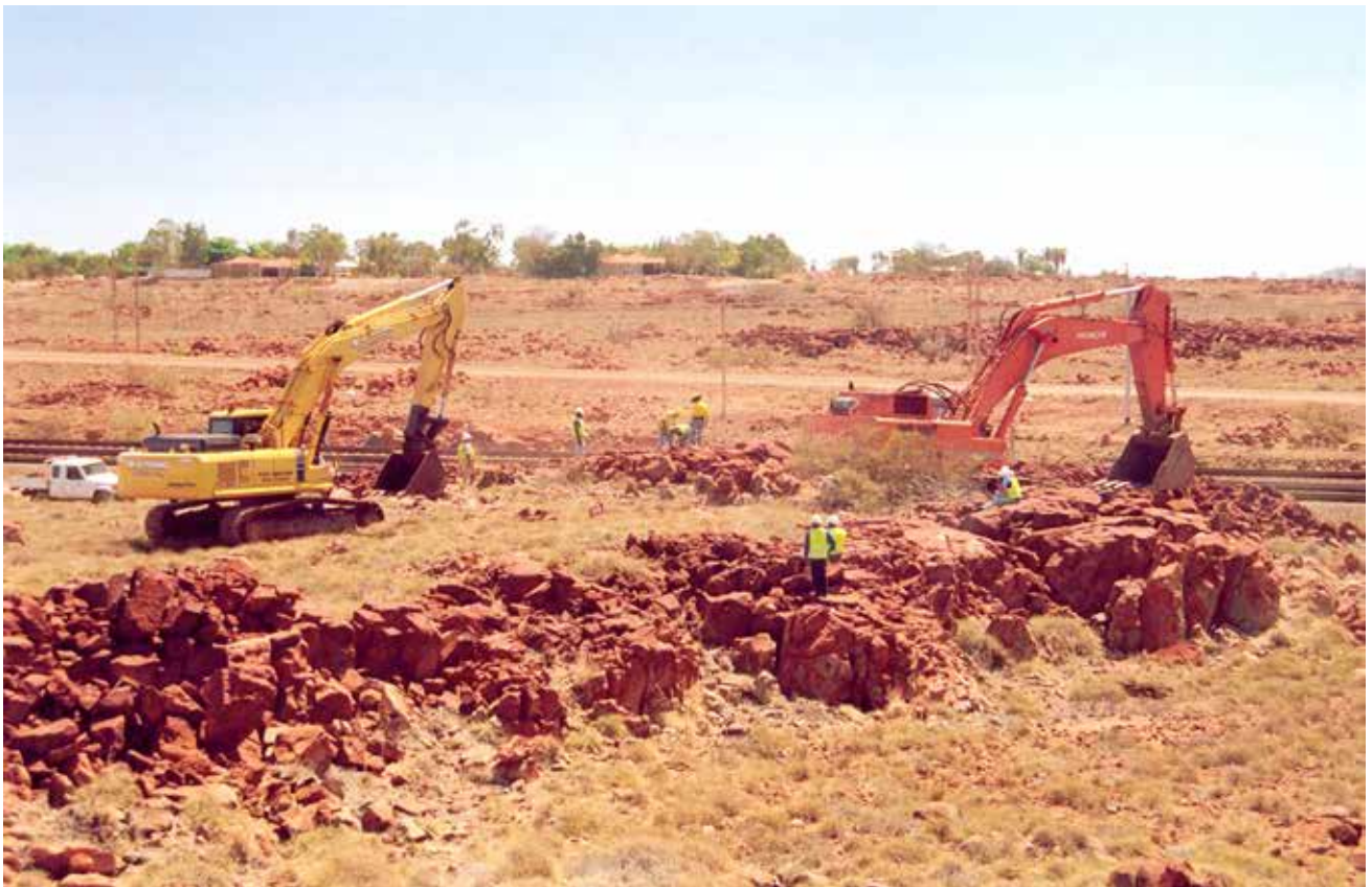
Figure 23. Construction work along the Rio Tinto rail line in May 2004 with Aboriginal custodians watching to ensure that activities do not impact petroglyphs. Dampier houses in background. Source: Photograph KJM.
